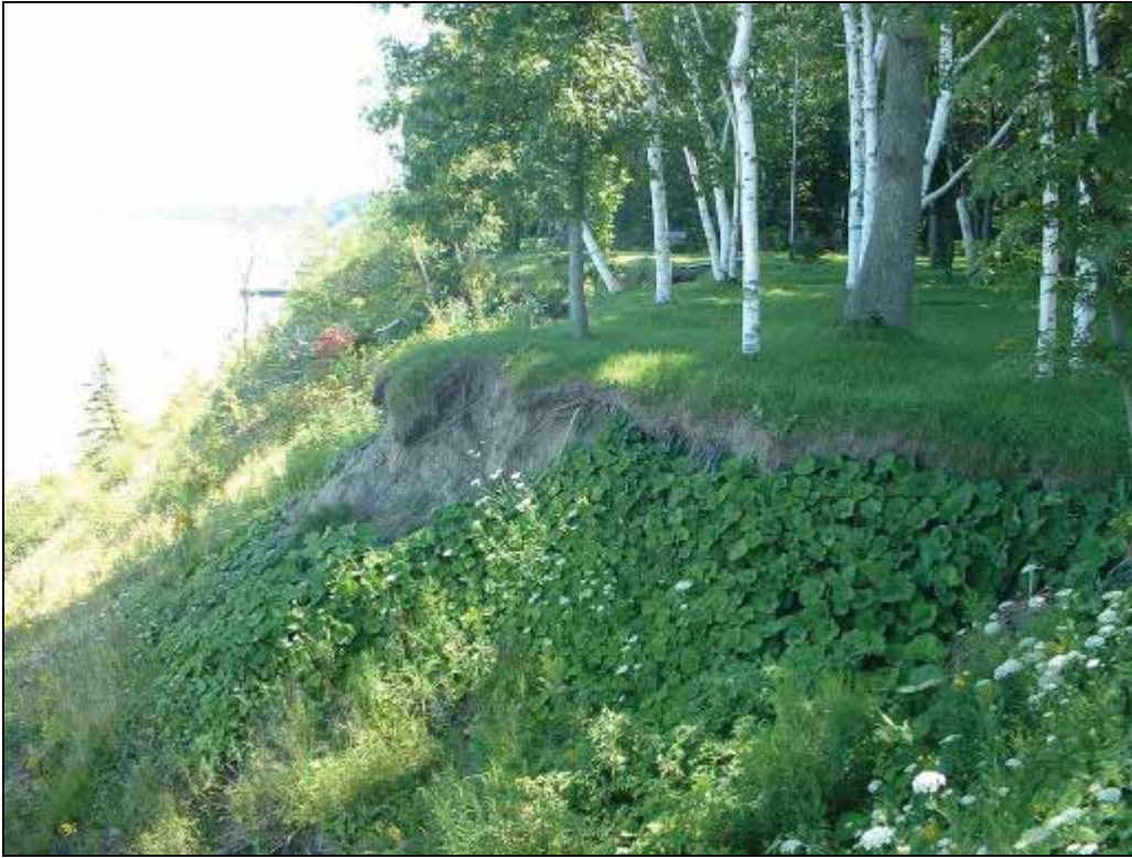
Figure C- Bank slumping in Block 1 (transects 583-586) Personal communication with landowners revealed that a 2004 rain event caused extensive top of slope sloughing 2004- St. Clair Region Conservation Authority
