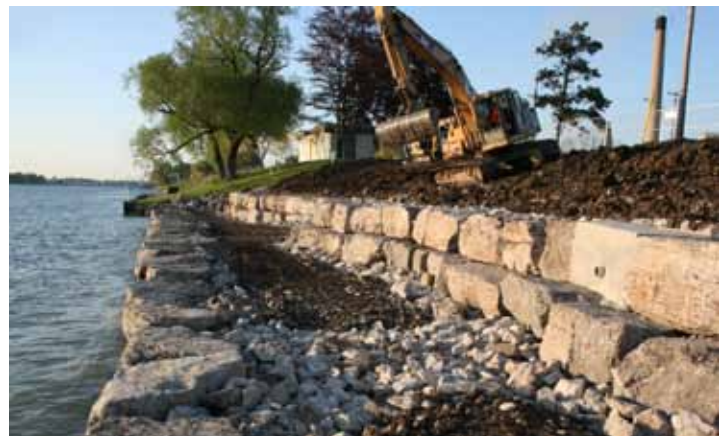
This innovative construction design provides for effective shore protection. Incorporated into the design is a planting pod which enhances shoreline habitat for fish and wildlife.
