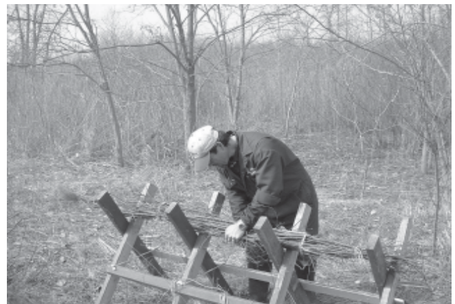
A fascine is a bundle of live cuttings that is placed into a trench along the streambank and grows to provide vegetative cover and stability to the slope. Cuttings are taken during the dormant season from shrubs of dogwood and willow.
