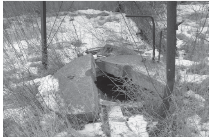
Before - an unused well that may contribute to direct groundwater contamination.
