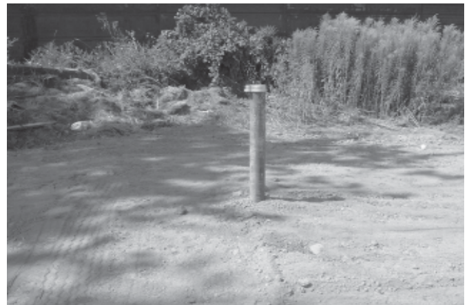
After - Repaired well with an extended casing 16" above finished level with a proper well head cap.
