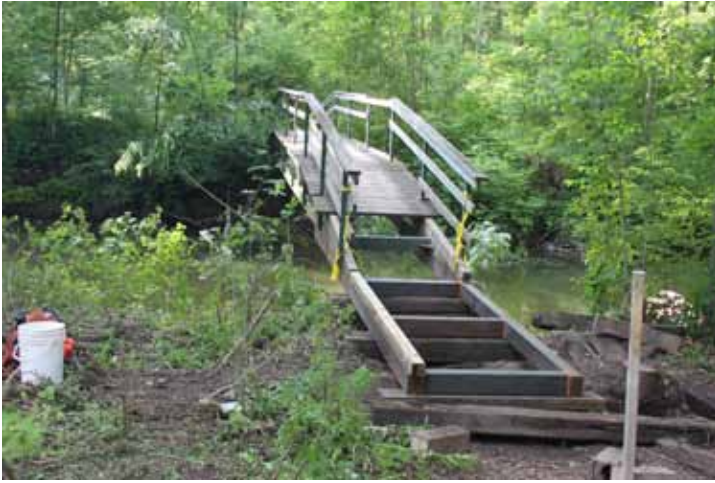
Major repairs to the trail bridge crossing the Sydenham River at the Strathroy Conservation Area were undertaken. An eroding stream bank threatened the integrity of the bridge. The bridge was lengthened and new approaches were installed.
