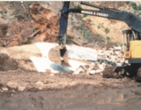
Erosion access allowance provides a route for machinery to undertake periodic repairs as well as emergency vehicles
