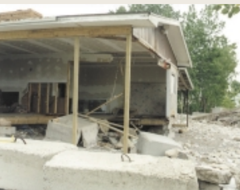
Flooding, wind and wave action damage to property on Lake Erie
