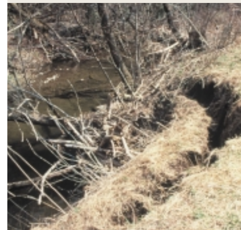
River bank erosion
