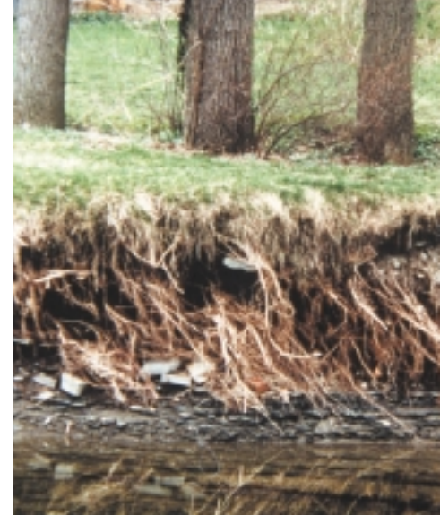
Eroding river bank
