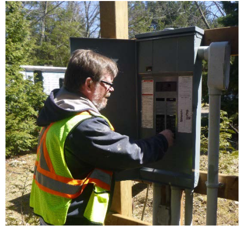
New hydro panel
