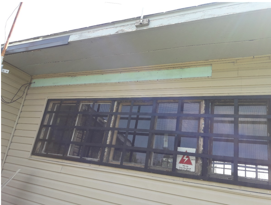
Siding and Fascia missing from building
