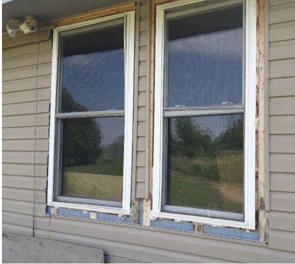
Trim missing around windows and plywood coming off of wall
