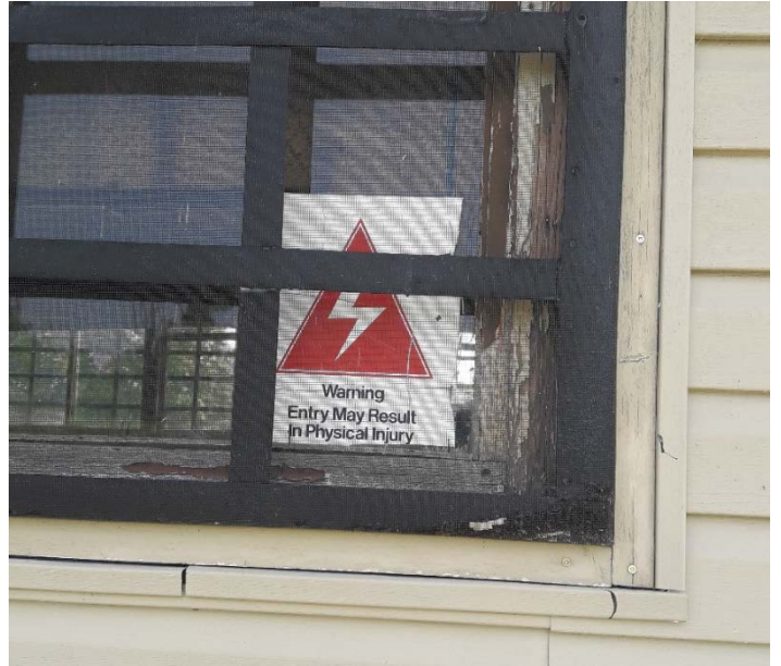
This sign is present in all windows
