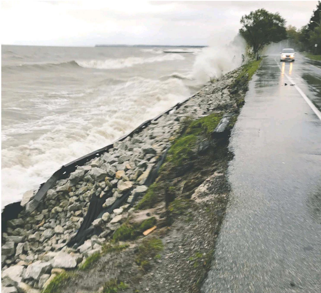
Erosion has forced the closure of a section of Old Lakeshore Road, city officials say. SUPPLIED
