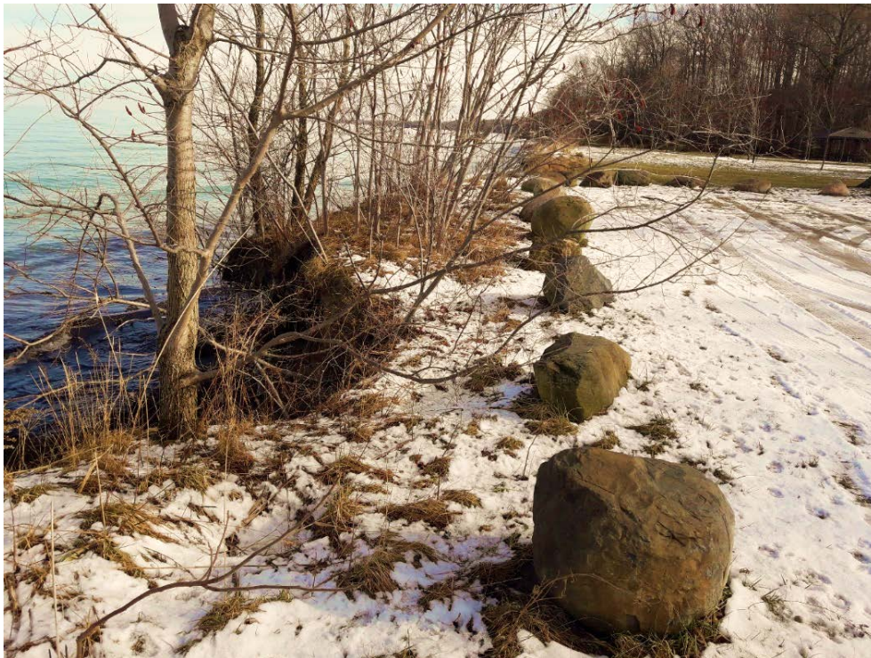
Erosion east of the ramp is approaching the parking lot.
