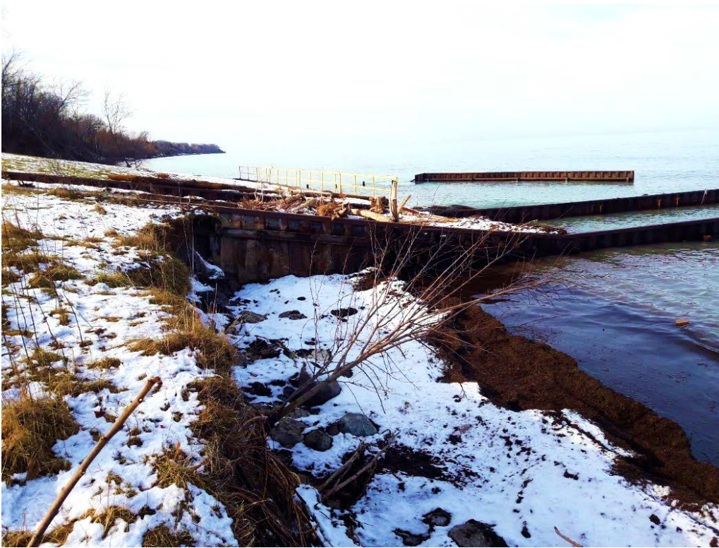
Erosion exposing the steel sheet wall that supports the boat ramp.
