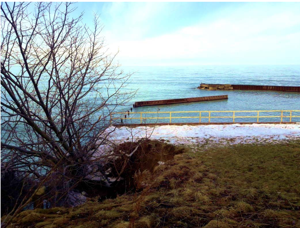
Erosion from the west is moving around the ramp protection.
