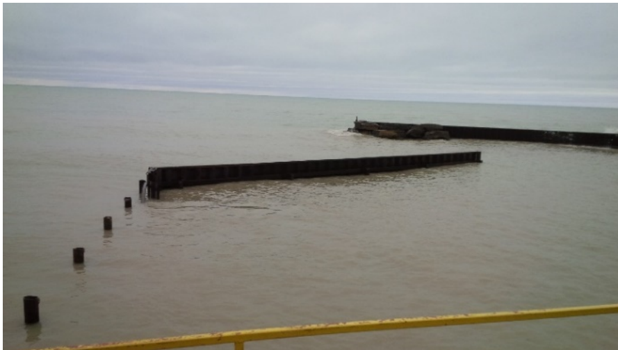
Damage to Groyne
