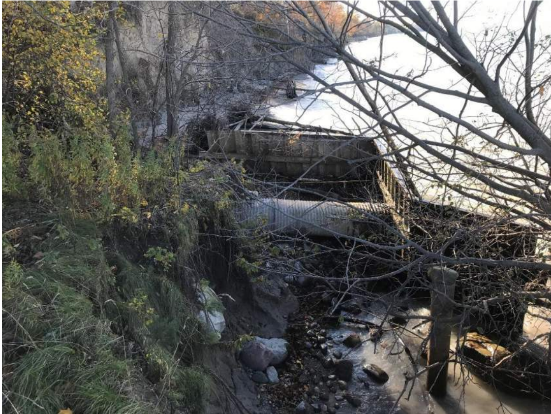
Photo 19- Erosion behind South Seawall Extension
