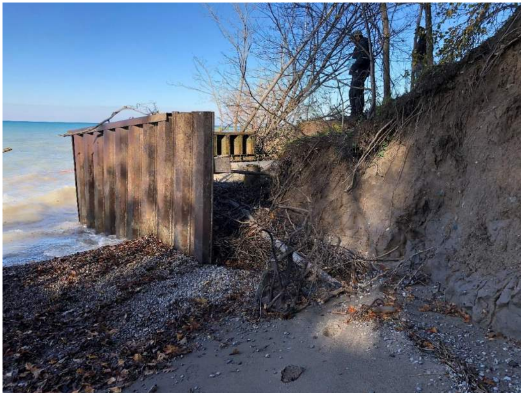
Photo 20- Erosion behind South Seawall Extension
