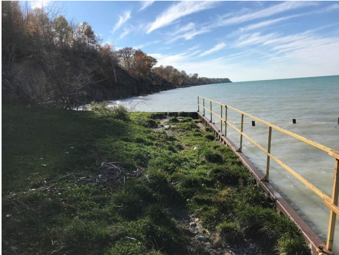
Photo 13- Erosion of Bank Along South Retaining Wall
