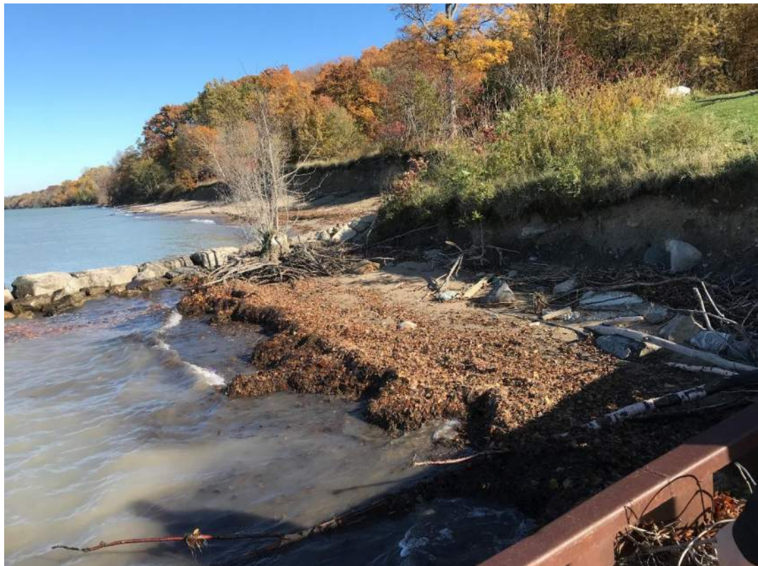
Photo 8- Erosion of Banks East of Boat Ramp
