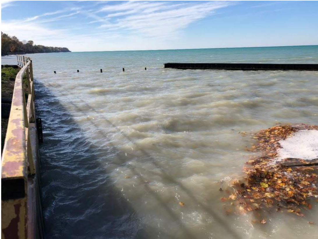
Photo 11- Missing Groyne Wall, Looking from Boat Ramp
