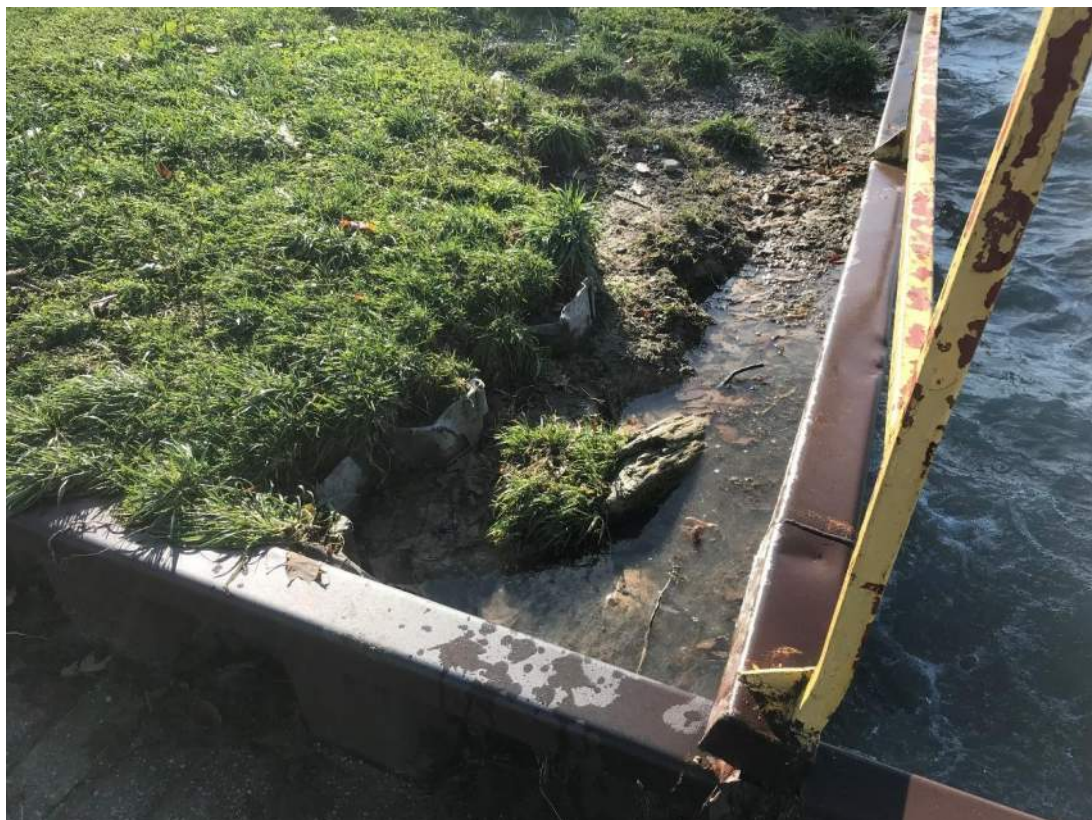
Photo 12- Erosion in Bank at South Retaining Wall, Note Buried Sheet Pile Wall
