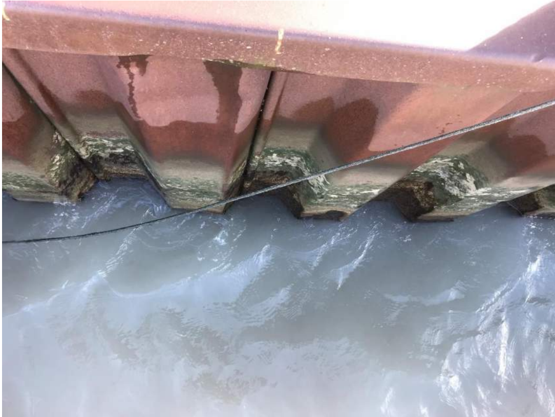
Photo 15- Staining on Sheet Pile of South Retaining Wall
