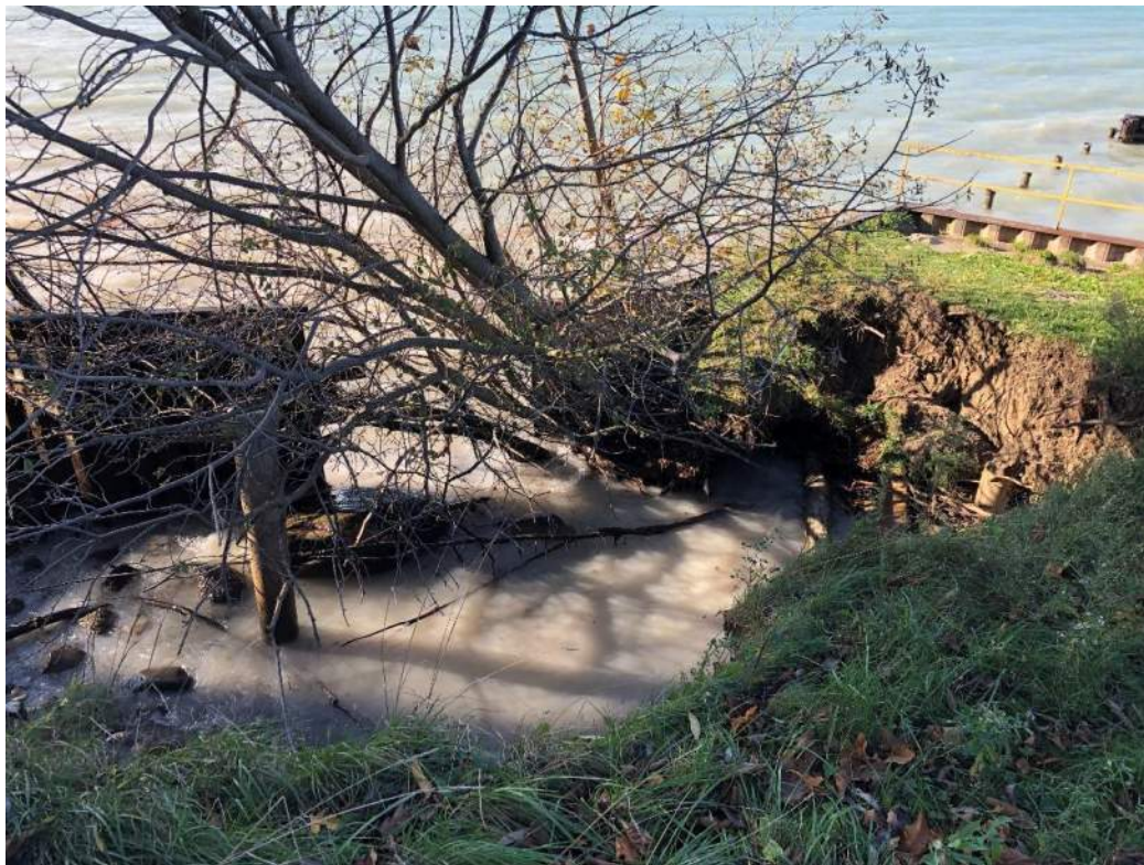
Photo 16- Erosion of Bank behind Groyne Wall and South Seawall Extension
