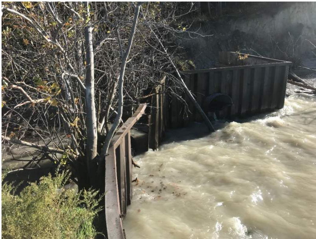
Photo 18- South Seawall Extension and Missing Segment of Groyne Wall
