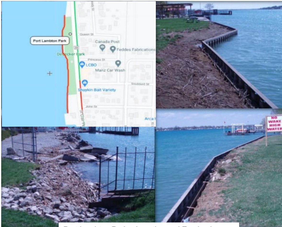
Port Lambton Park – Location and Erosion issues
