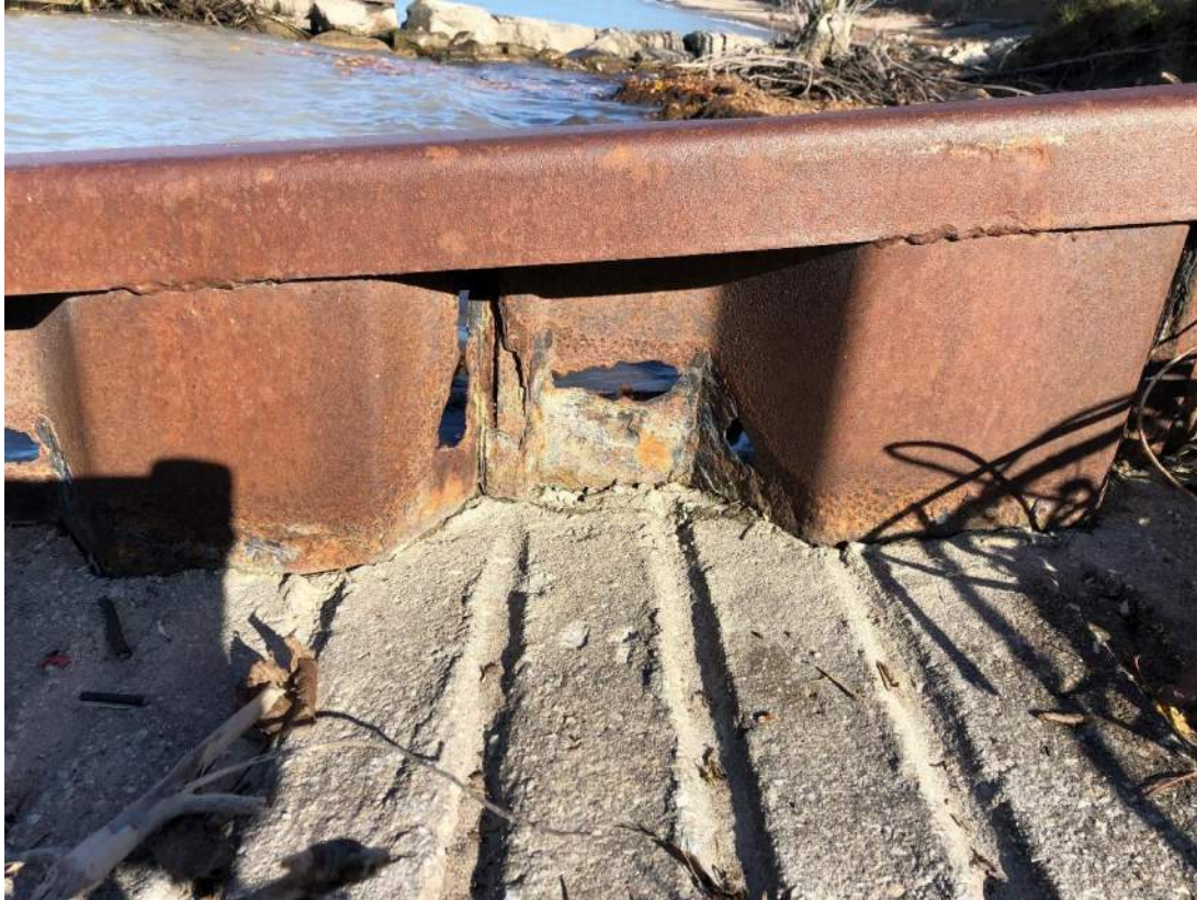
Photo 5- Corrosion with Section Loss and Perforations, Boat Ramp Sheet Pile
