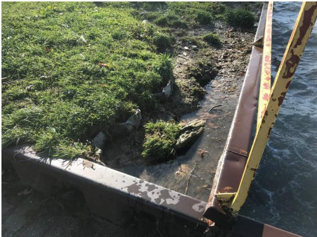
Photo 12- Erosion in Bank at South Retaining Wall, Note Buried Sheet Pile Wall
