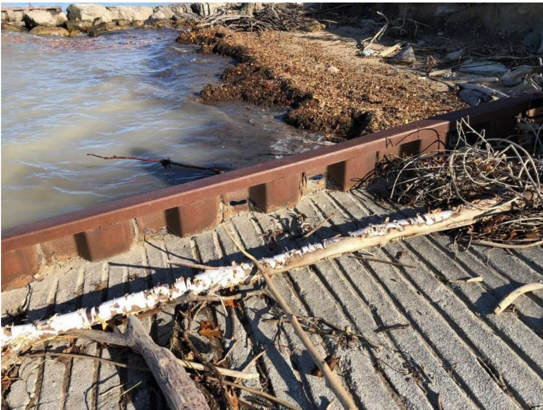
Photo 4- Corrosion of Sheet Pile Wall at Boat Ramp
