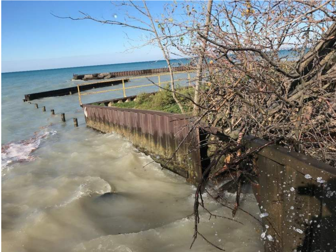
Photo 17- Missing Segments of Groyne Wall
