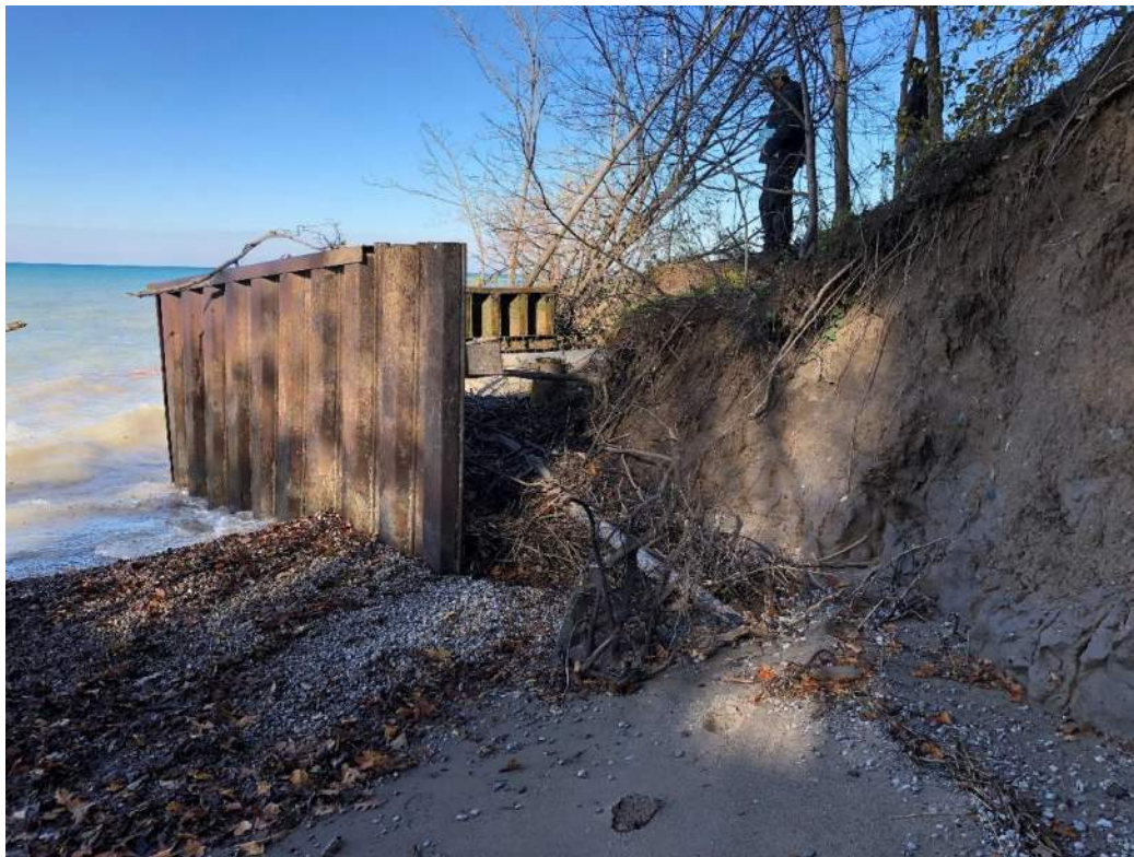
Photo 20- Erosion behind South Seawall Extension
