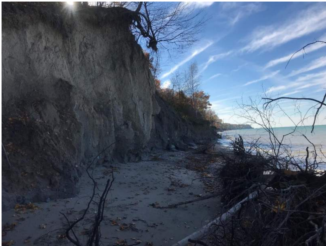
Photo 22- Erosion of Bluff West of Boat Launch
