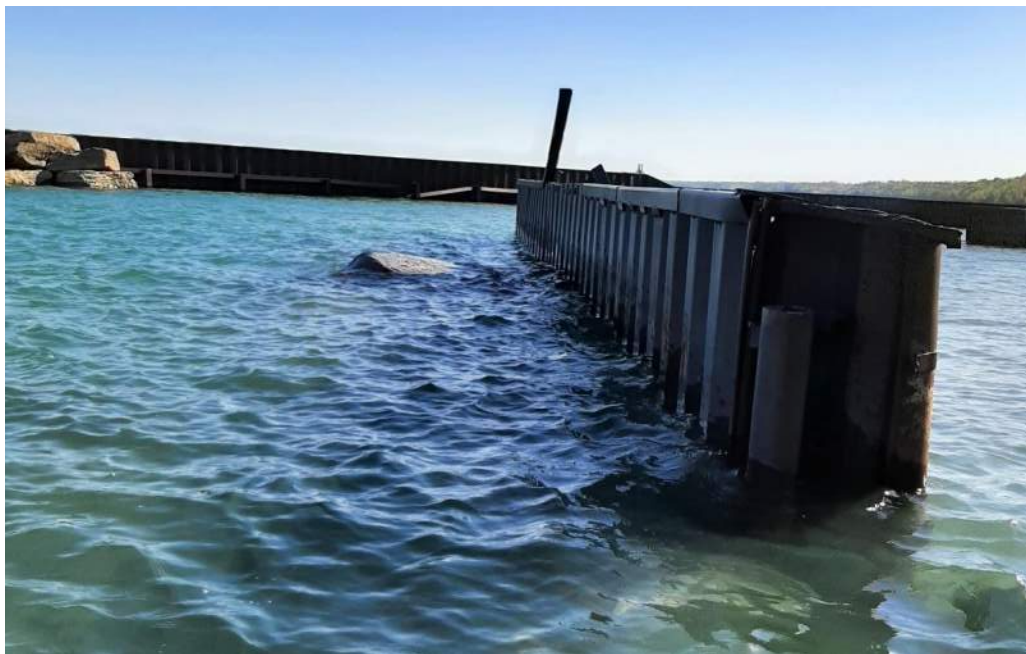
Photo 30- West Breakwater looking East – note bent pile cap on West Breakwater and loose Waler on Northeast Breakwater in background
