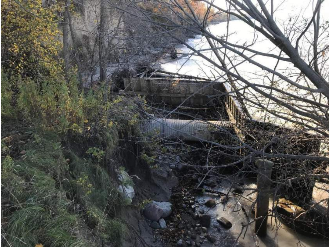
Photo 19- Erosion behind South Seawall Extension
