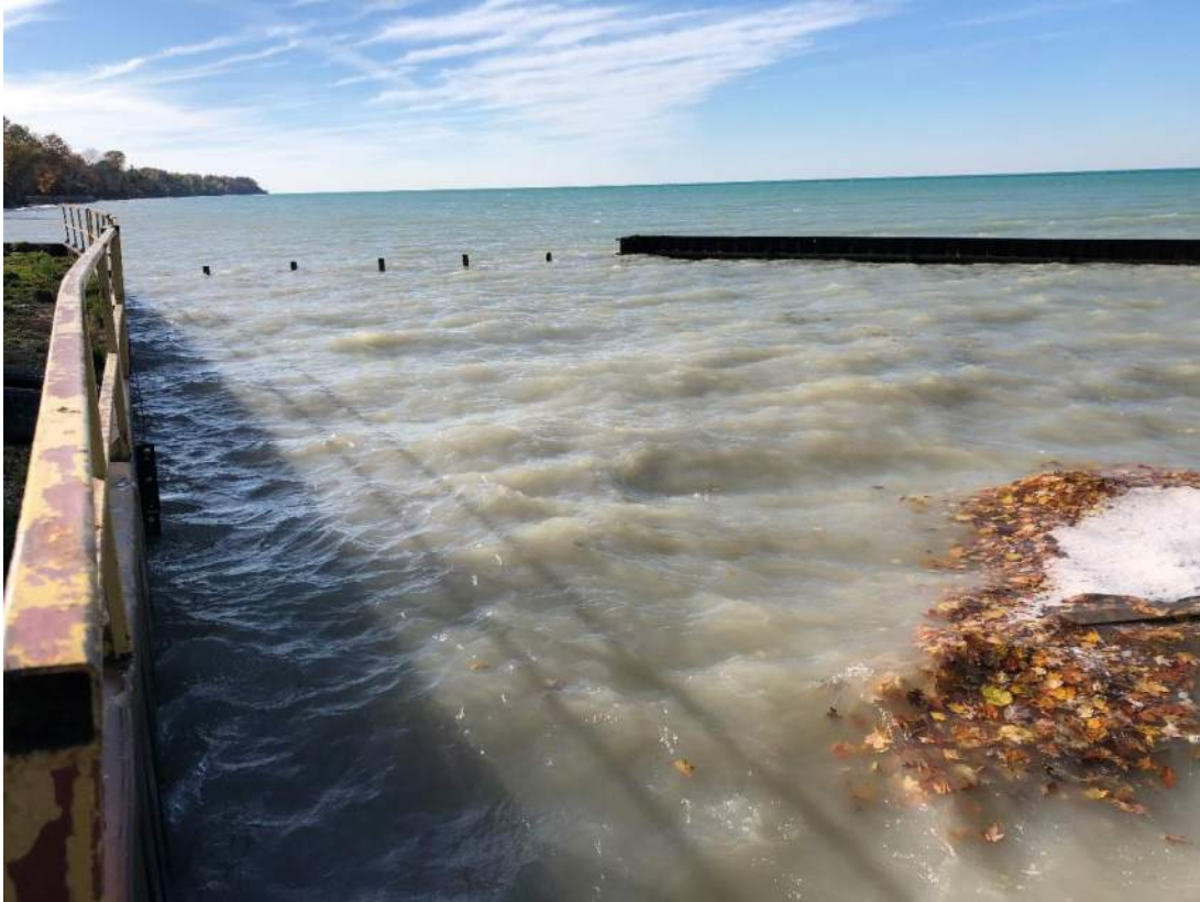
Photo 11- Missing Groyne Wall, Looking from Boat Ramp
