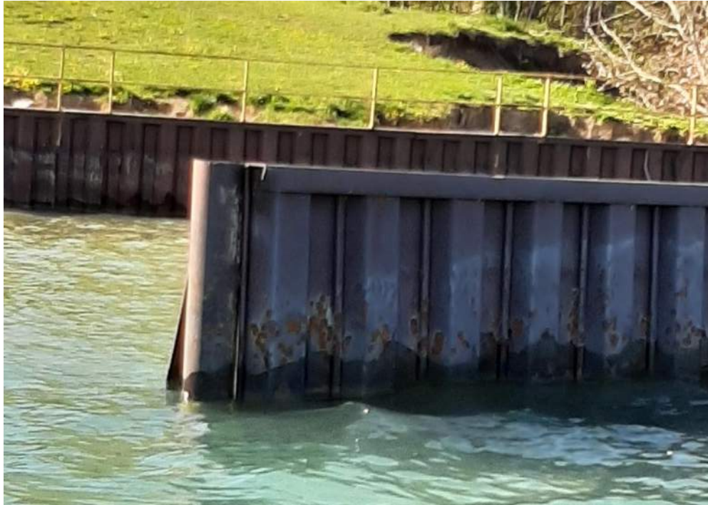
Photo 29- Corrosion of sheet pile above waterline at West Breakwater
