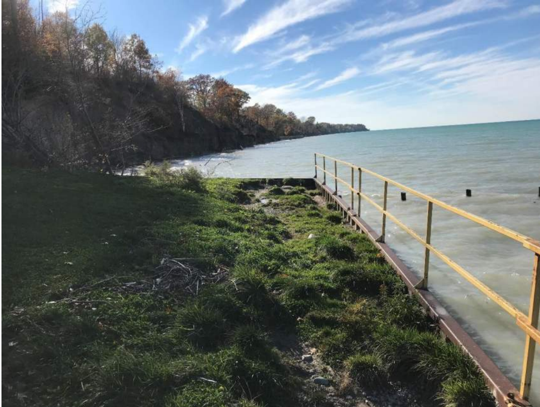
Photo 13- Erosion of Bank Along South Retaining Wall
