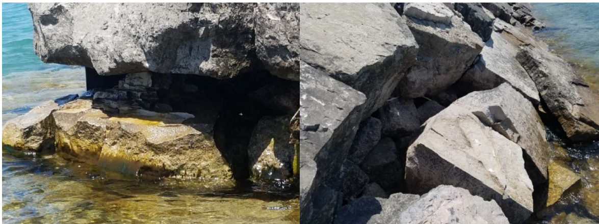
Failed sections of armourstone revetment along LAWSS shoreline
