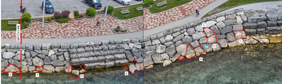
Extent of failure along LAWSS shoreline
