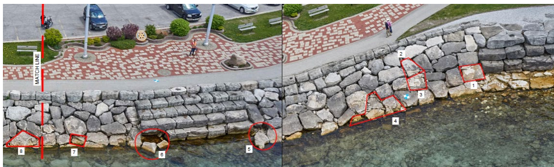
Extent of failure along LAWSS shoreline
