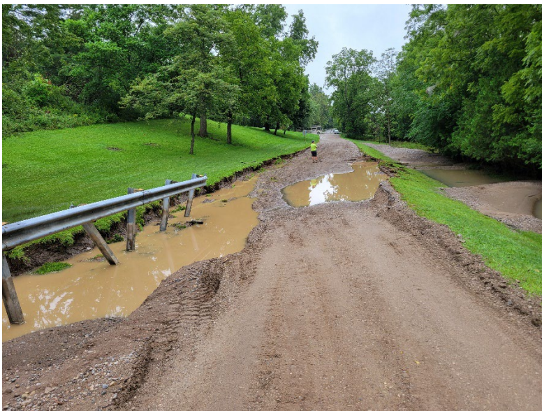
Above image is of the road damage when the water receded
