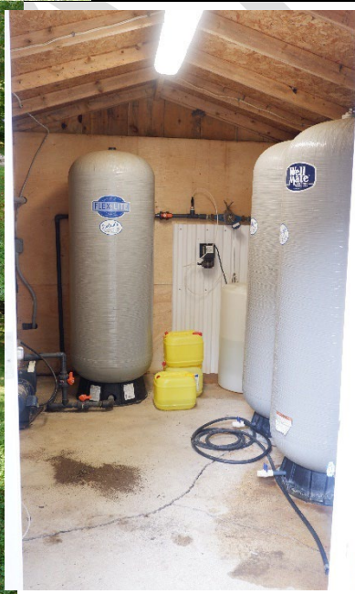
Chlorinated water treatment system located in pump house
