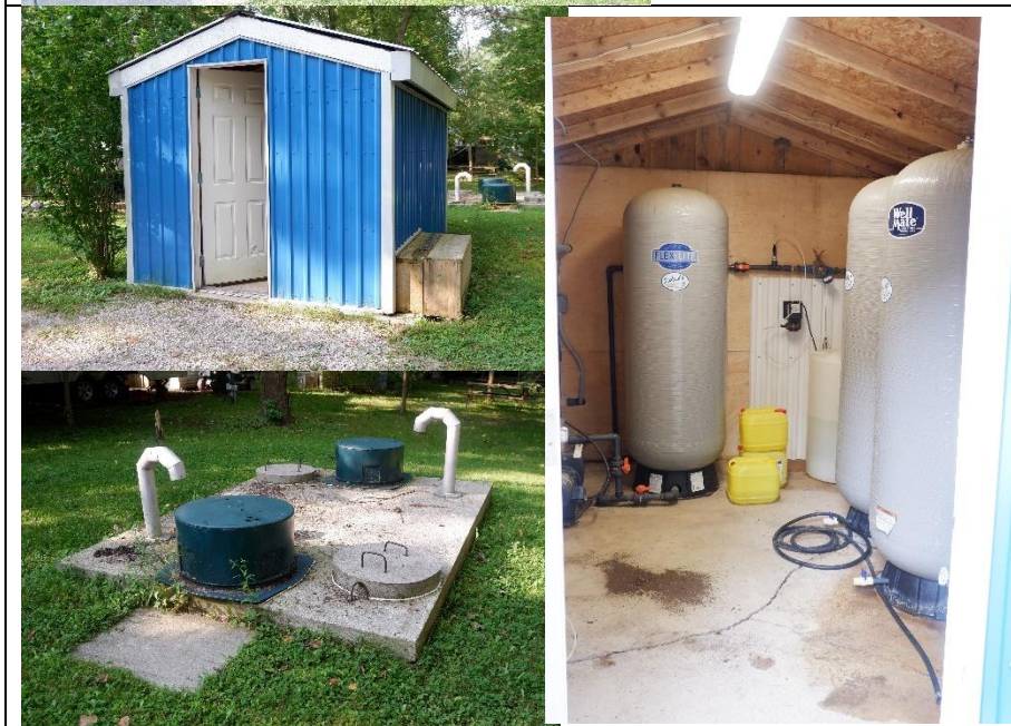
Chlorinated water treatment system located in pumphouse
