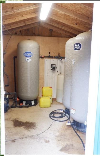
Chlorinated water treatment system located in pumphouse
